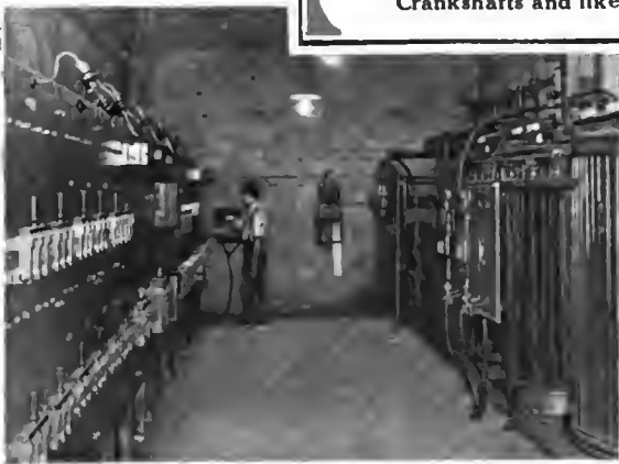
B—The Entire Plant is Operated by Electric Motors. This is a View of the Main Switchboard and the Battery of Transformers from which the Electric Current is Taken
